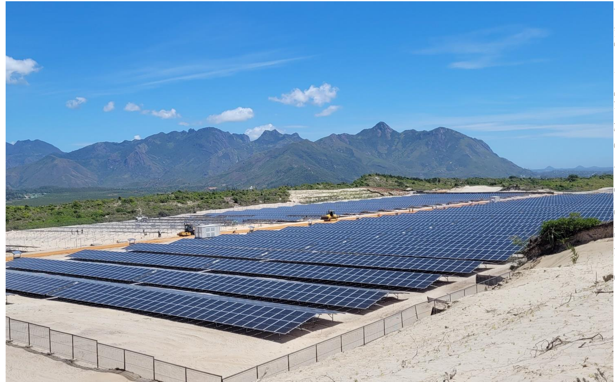
CBE QIT Madagascar Minerals (Rio Tinto) Project Fort Dauphin, Madagascar 8MW solar, 8.25MWh BESS
